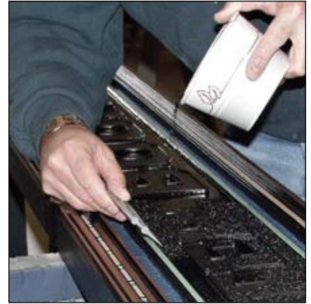
Normally I will do the osmalto (smaltz) work prior to the finish painting but in this case the area was separated and trapped quite well and I saw no need to stop my rhythm of work. A bath of tinted epoxy is brushed into the receiving area and black smaltz is poured over the still wet surface and allowed to cure before dumping off the excess. While pouring the smaltz I used a long squeegee to act as a dam to help keep it contained within the targeted area.
